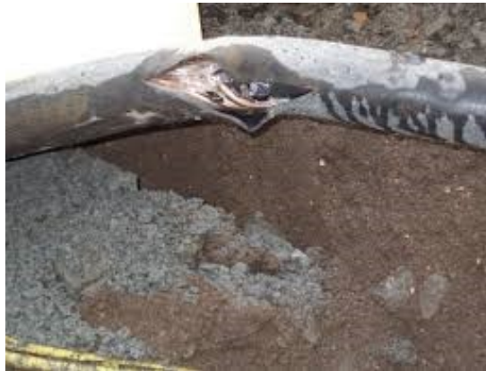
Figure 1.2 Excessive Bending as a part of Mechanical Damage in Power Cable [2]
