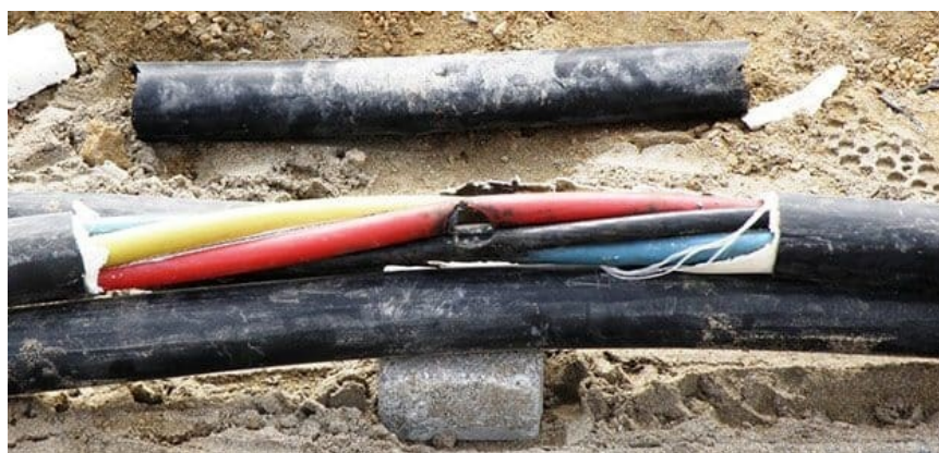
Figure 1.3 Electro thermal Damage in Cable [3]
